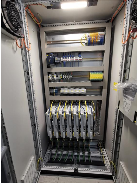
Hexapod amplifiers cabinet
